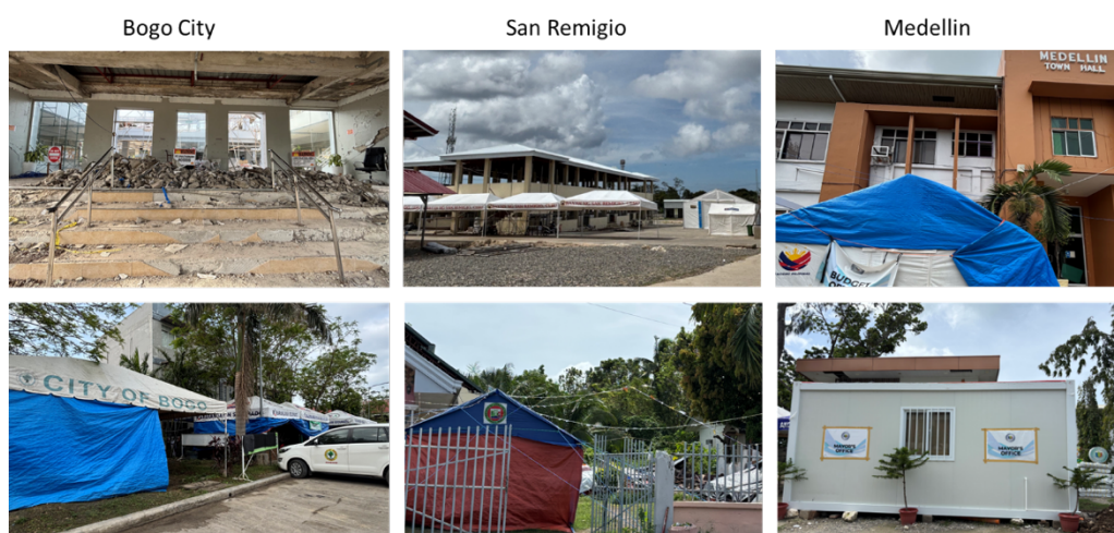
Figure 5 Damaged local government office buildings (above photos); tents and containers as temporary offices (below photos)
